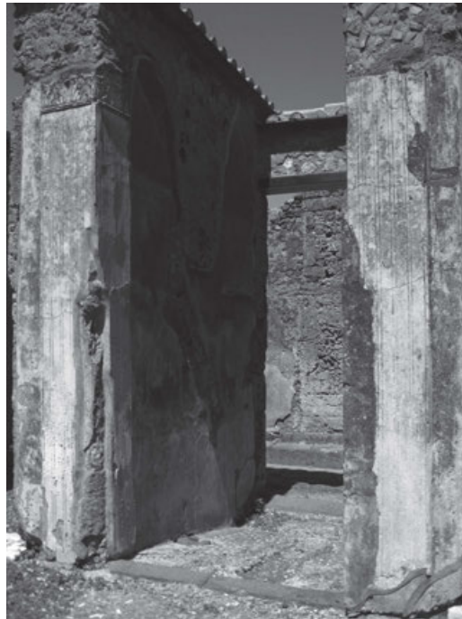
Figure 9: Inner entrance doorway of the Casa delle Danzatrici (VI.2.22), showing the wide, vertical plaster scars on the Fourth Style fluted, stuccowork jamb pilasters. The scar on the south jamb (right) has been filled with modern plaster. (Photo by the author)
