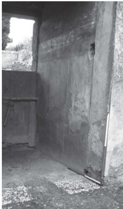
Figure 6: The west wall of the entrance passage in the Casa di Cerere (I.9.13), showing a hole in the wall base for a wooden sill, and a larger hole at 2.10m height for a wooden transom. A plaster cast of the main, outer entrance door can be seen in the background (left). (Photo by the author)
