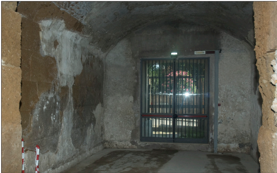
Figure 3: One of a series of rooms on the north side of the Capitoline substructio , which may once have housed activities associated with the mint (Author's photo, 2009).
